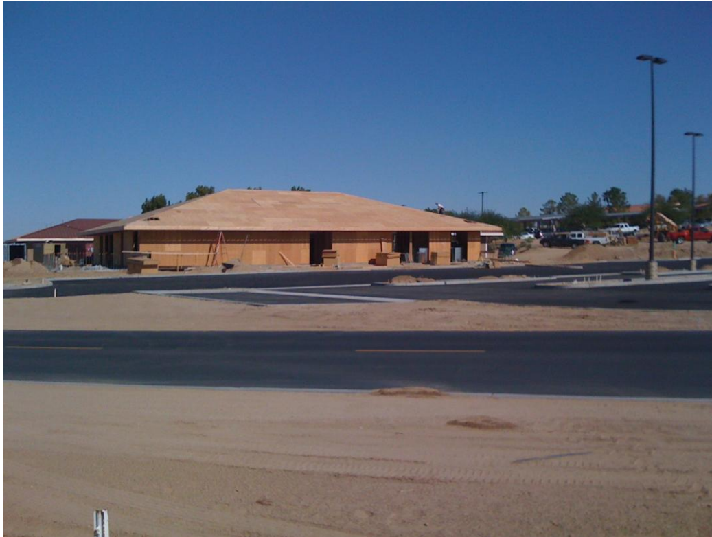
Photo Exhibit 1. Construction in the Remodel For Efficiency (RFE) Project north of Congressman Lewis Drive on 24 September 2010.
