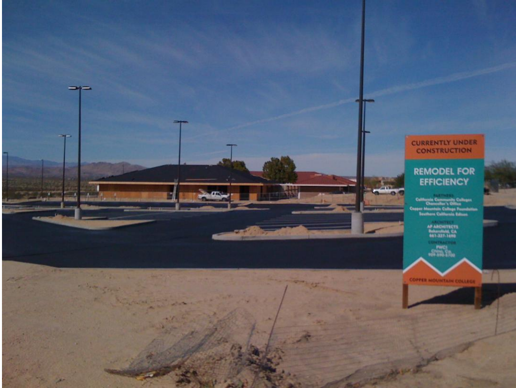
Photo Exhibit 1. Construction in the Remodel For Efficiency (RFE) Project north of Congressman Lewis Drive on 29 October 2010.
