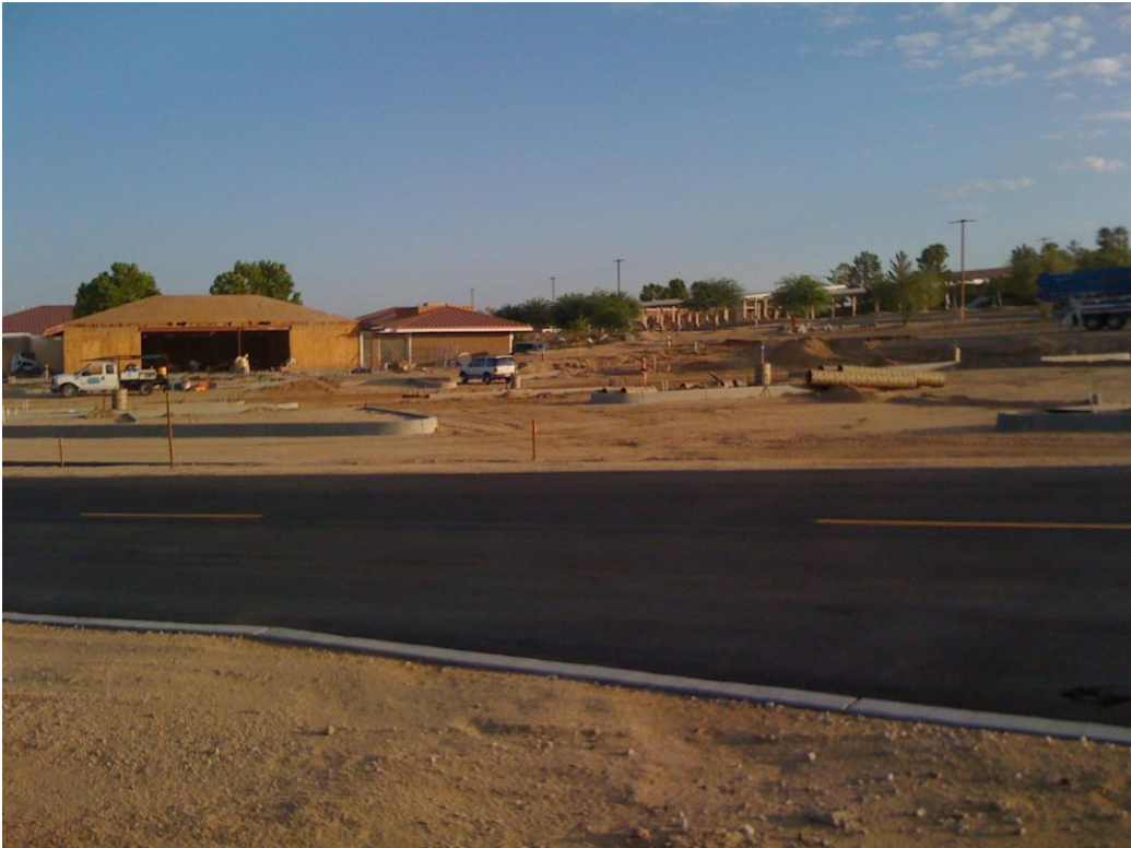
Photo Exhibit 2. Construction in the Remodel For Efficiency (RFE) Project north of Congressman Lewis Drive, 30 July 2010.
