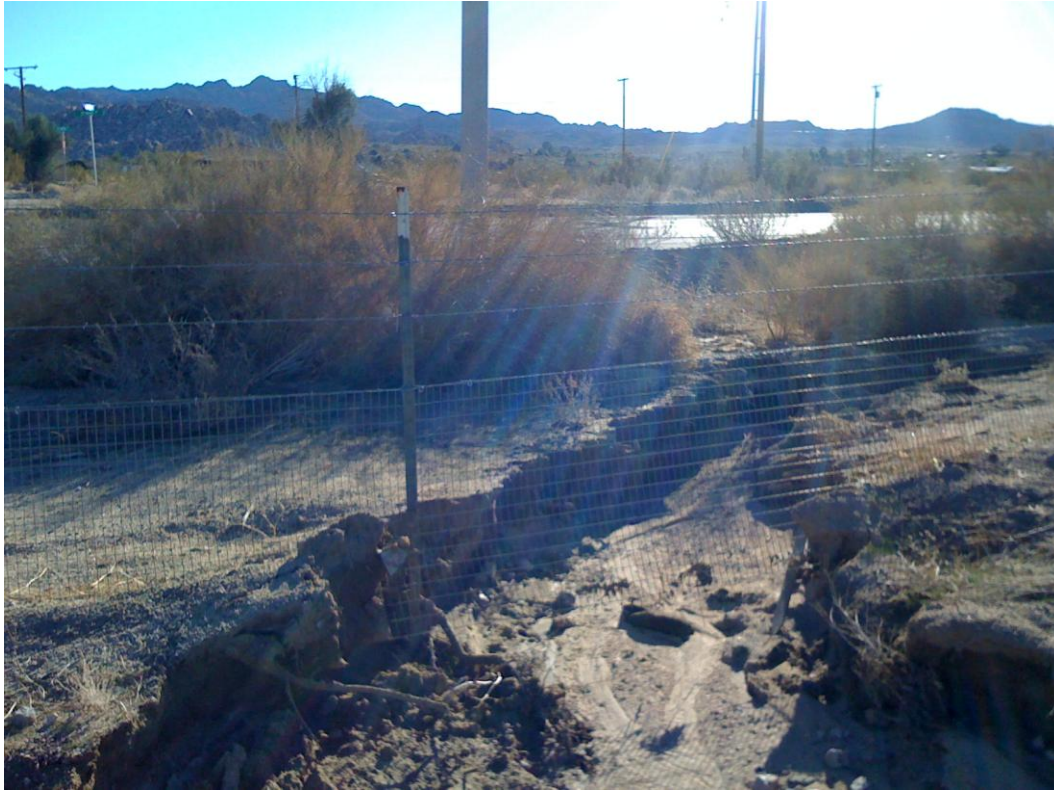
Photo Exhibit 1. Erosion due to rain water undercutting southern TA fenceline, 27 December 2010.
