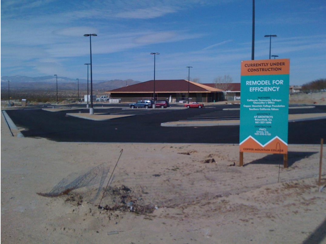
Photo Exhibit 1. Project site (IA) for the Remodel for Efficiency (RFE) Project at Copper Mountain College, 25 February 2011.
