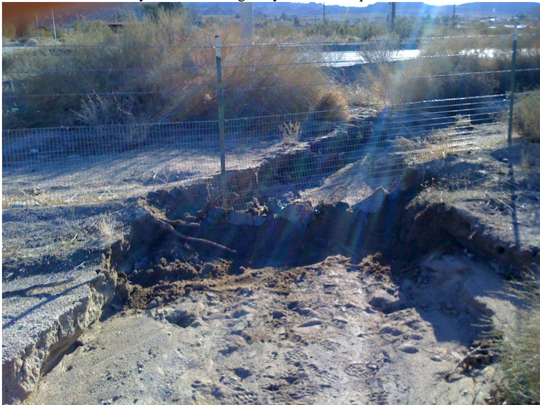
Photo Exhibit 2. Temporary repair of gap under TA fence using rocks, 27 December 2010.
