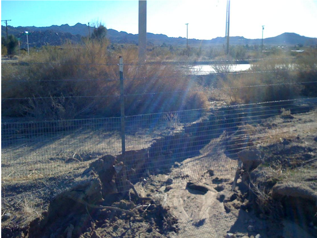
Photo Exhibit 1. Erosion due to rain water undercutting southern TA fenceline near intersection of Twentynine Palms Highway and Mile Square Road, 27 December 2010.
